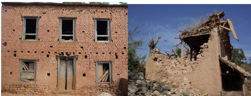
Figure 2. Difference of building damages between house materials Bricks and woods (left) and Muds and rocks (right)
